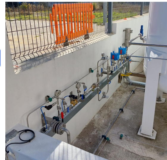
H2 pressure regulation and odorization at Gestene
