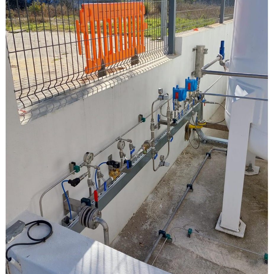
H2 pressure regulation and odorization at Gestene
