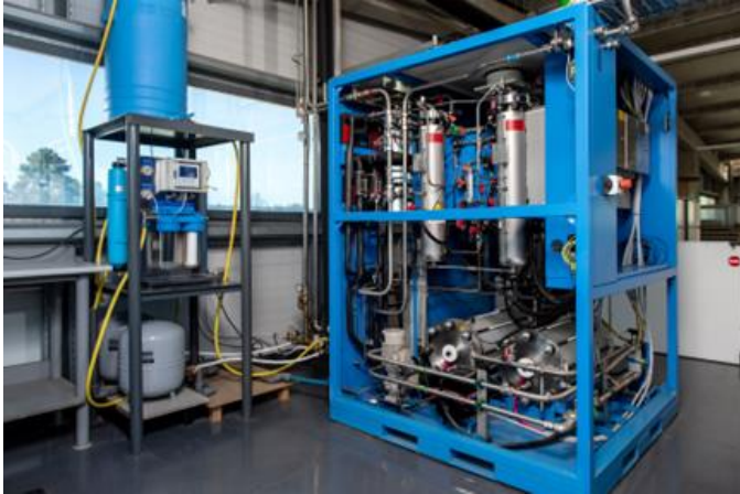
Electrolyser at Gestene
